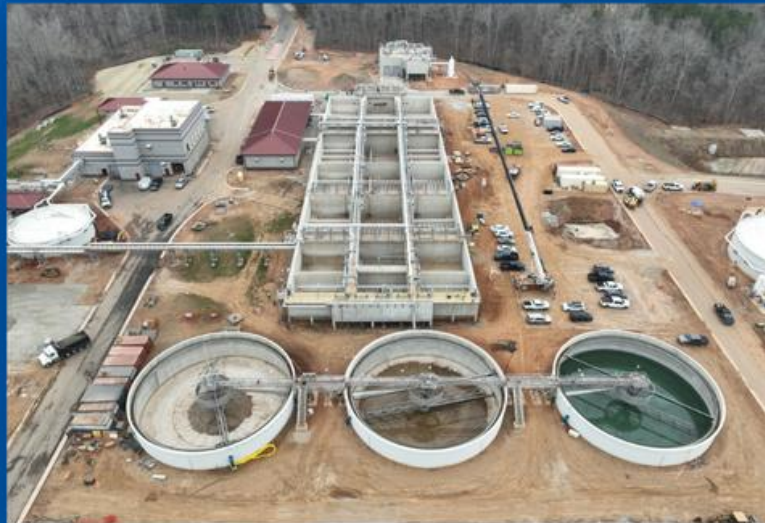
Sam's Branch Water Reclamation Facility
