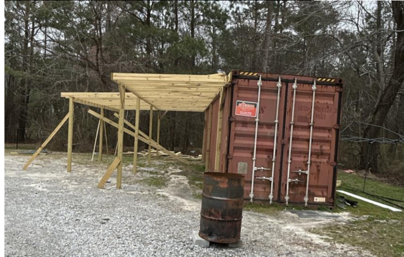
Work Without a Permit
