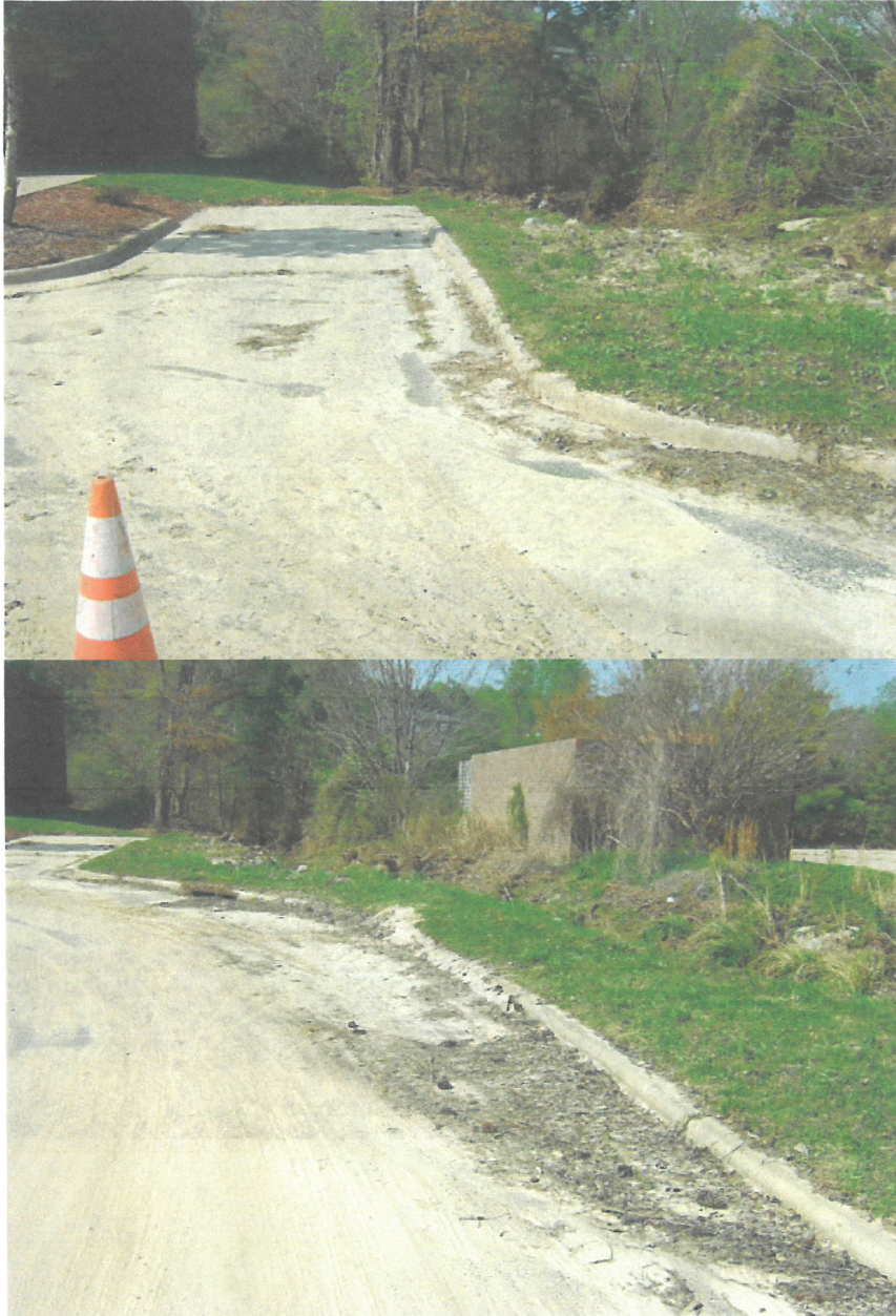
March 2010 flooding debris.
