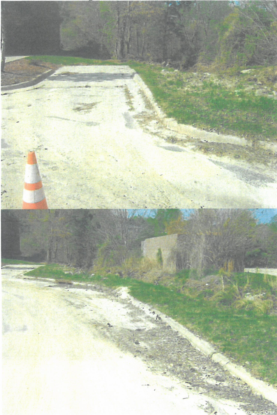
March 2010 flooding debris.
